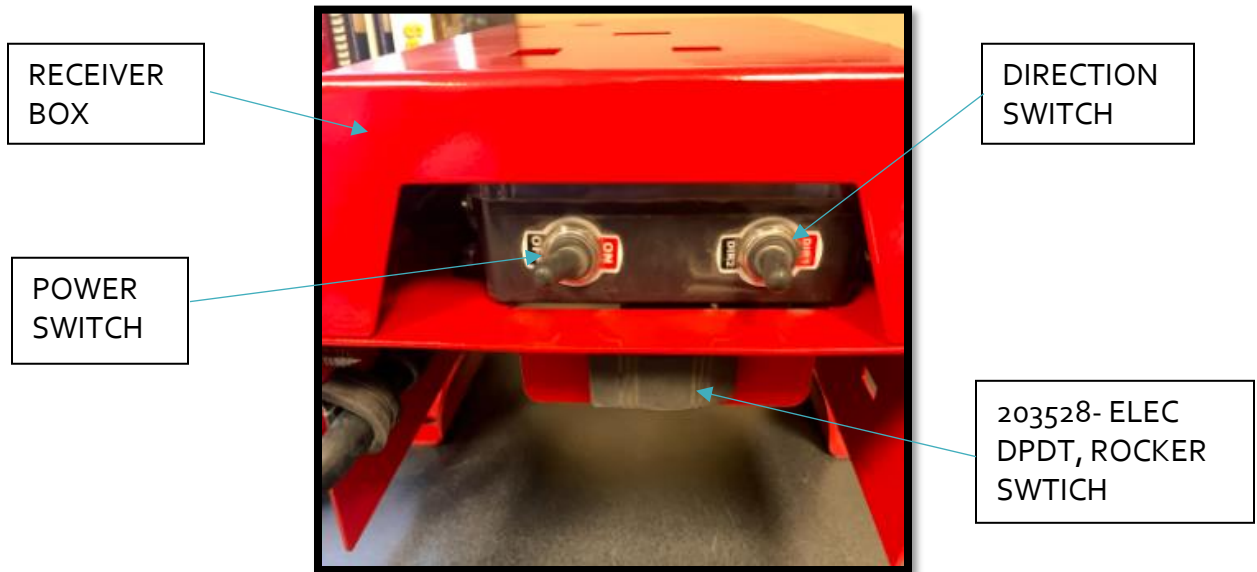
Figure 25: Power Swing Receiver Box
